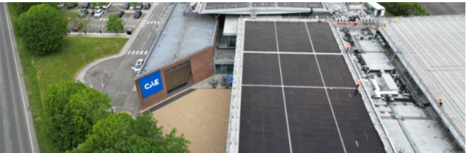
CAE’s Burgess Hill training centre is now powered by nearly 2,000 solar panels, providing about 20% of its annual electricity.
